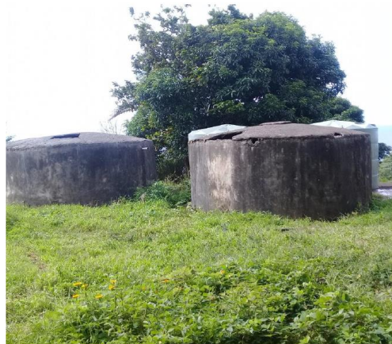
The old storage tanks (22500L *2)
