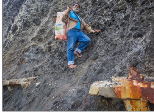
Above: Villager clings to side of cliff due to damaged walk-way and lack of railing (PC - Niki Kuautonga)
