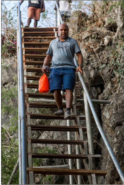
UNDP Analyst using staircase on footpath between Ipau & Herold Bay (PC - Niki Kuautonga)
